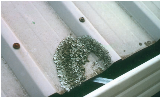
Figure 3: Photograph of lichen on a roof made from COLORBOND® steel.
