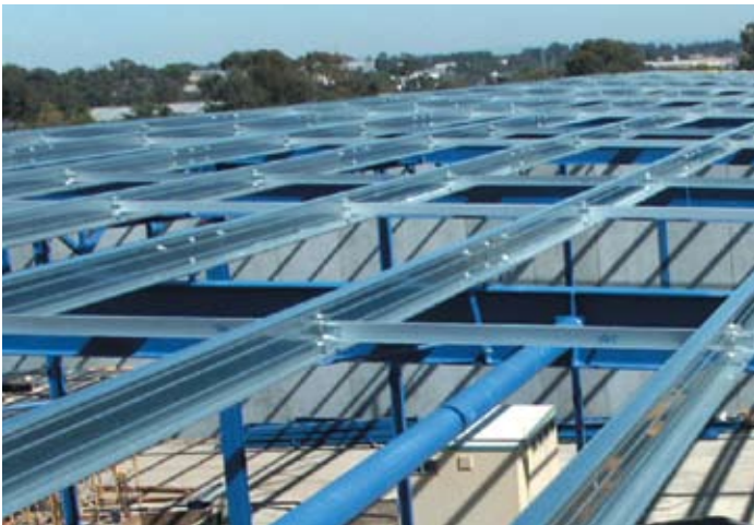
Galvanised steel purlins
