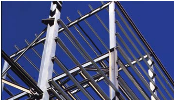
Galvanized steel purlins
